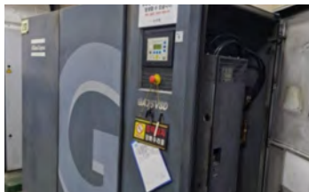
Operation of VSD(Variable Speed Drive) Compressors
